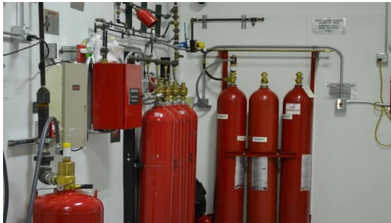
Figure 13: Fire Suppression System
